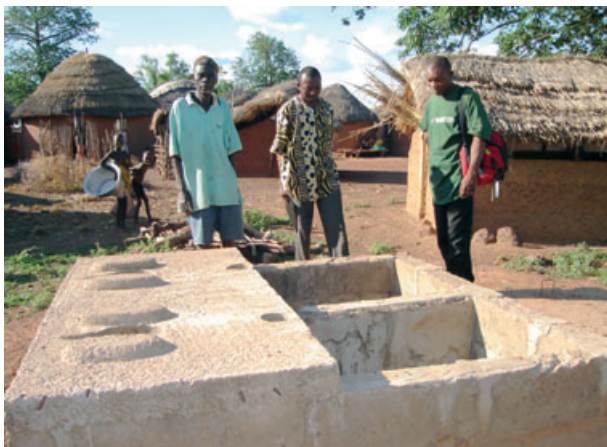
Figure 4 An unfinished compartment latrine. Construction had been halted for at least 1 year in 87.2% of all unfinished latrines observed. It is doubtful this latrine will ever be completed and used.
